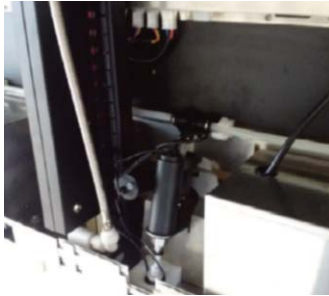
The 12v soap dispenser in-situ
